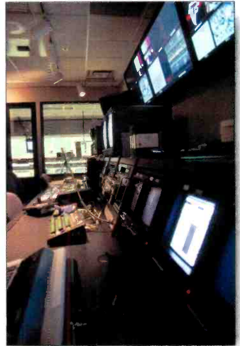
The Georgia Dome chose the Evertz MVP multivideo processor, with three Mitsubishi LCD monitors for display instead of a traditional monitor wall found in most control rooms.
