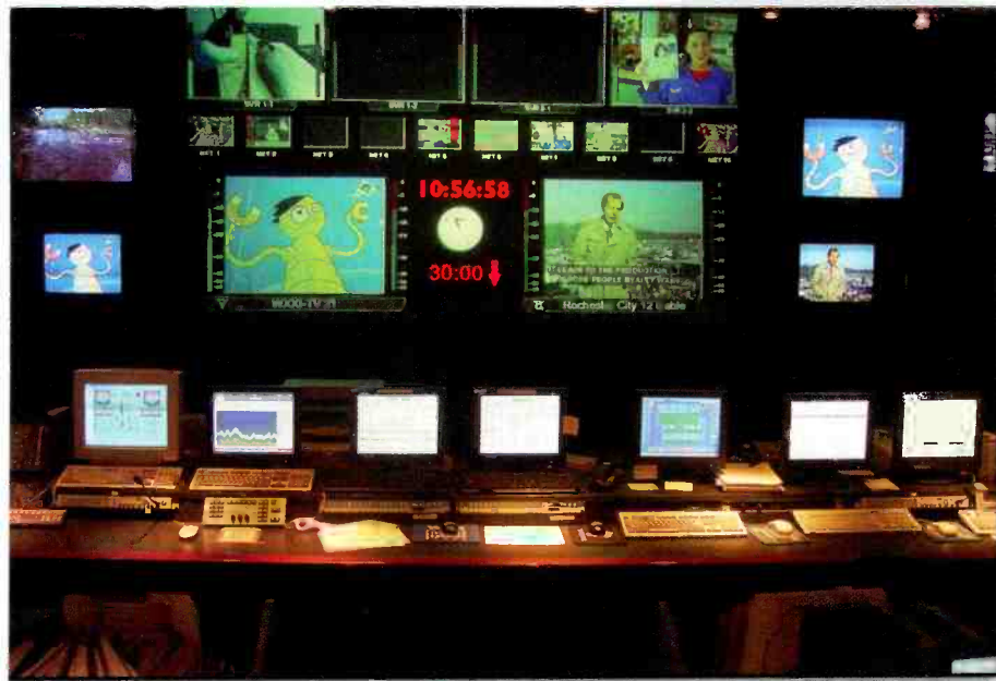
As program services and requirements change, this rear-projection "glass cockpit" monitor wall can recall multiple configurations of source monitoring.
