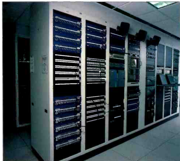
The TNT portion of the central equipment room is a designated area that allows for immediate action to any equipment problems.
