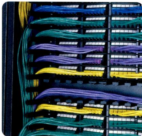
Integrator shown in cabinet
