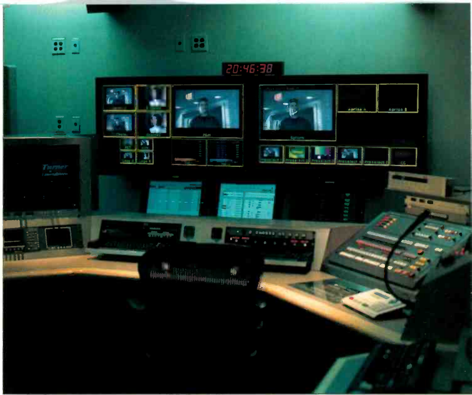
The test control room replicates the layout and design of a functioning BOC. This room provides a designated area to test and evaluate hardware and software in a simulated broadcast and media operations environment.
