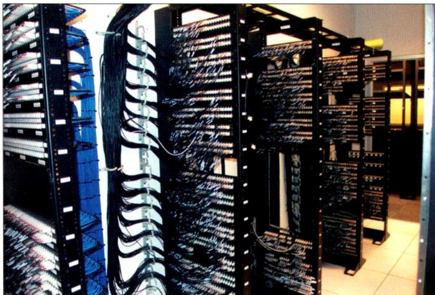
At WALA, Elco audio bulkheads were used in place of a normal patching system to facilitate system reconfiguration while avoiding the problems associated with patchbay corrosion.
