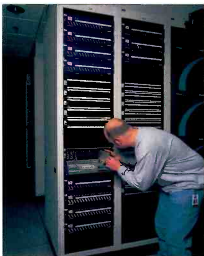
Maintenance engineer Chuck Armitage adds a module to one of the numerous Snell & Wilcox IQ Modular systems throughout the facility.
