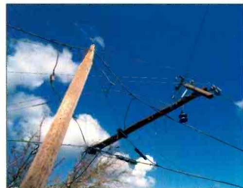
A snapped utility pole dangles helplessly after a storm. Don't let your station suffer the same fate.
