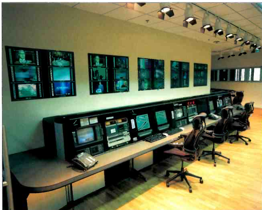
The incoming TOC is generally dedicated to the reception of live feeds. Operators here coordinate satellite uplinks and feed signals to the appropriate BOC with a Thomson Grass Valley Trinx router.
