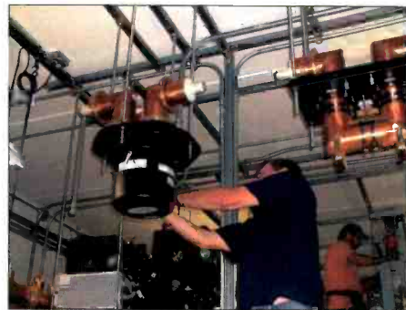
Stations are responsible for the safety of personnel working in high-RF environments, as well as for the safety of members of the general public. Photo courtesy Wisconsin Educational Communications Board.
