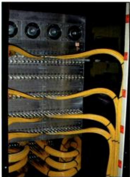
Netcom's PatchAmp, shown above, allows facilities to reduce their wiring requirements.
