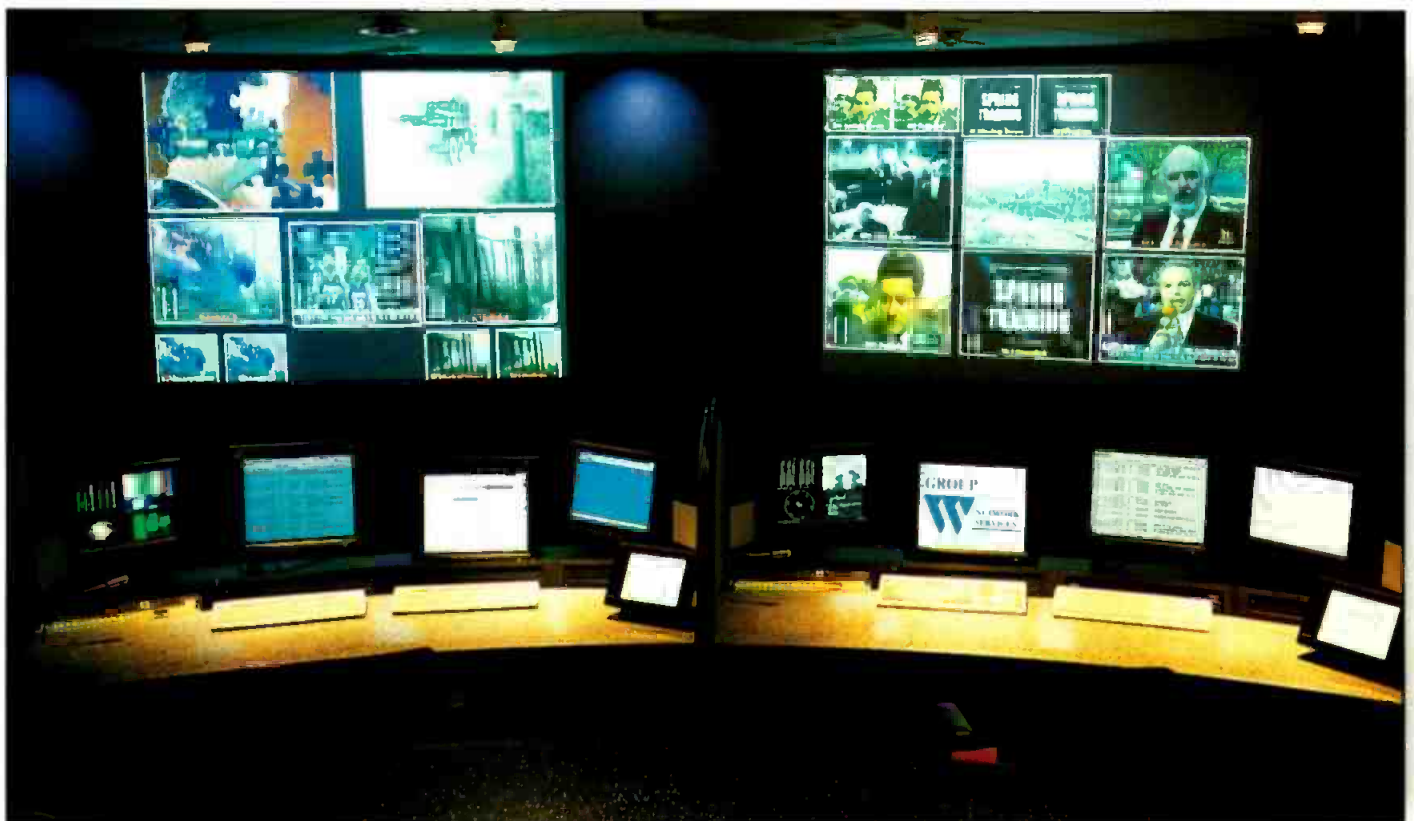
The master control facility at Harbor Plaza serves strictly as a monitoring station for automation systems in both facilities. Besides the monitors and projectors, there is no other electronic equipment in the control room.
