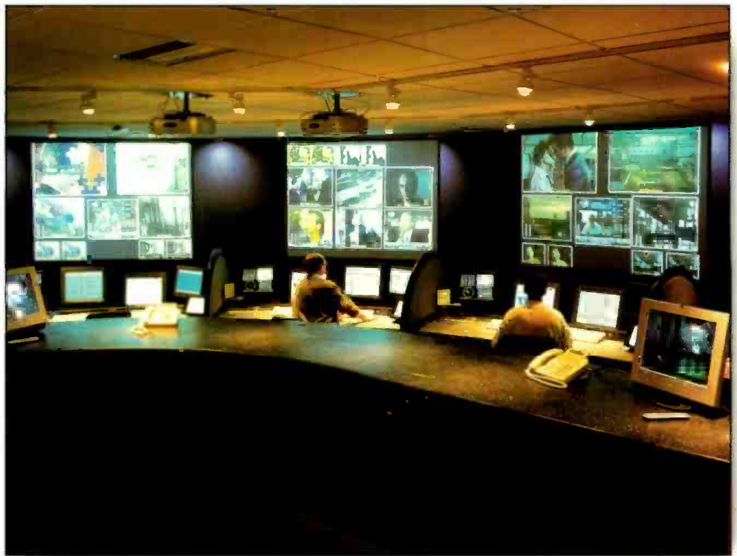
In GWNS' master control facility, five master control stations each handle four networks, monitoring four video images for each network's signal path.
