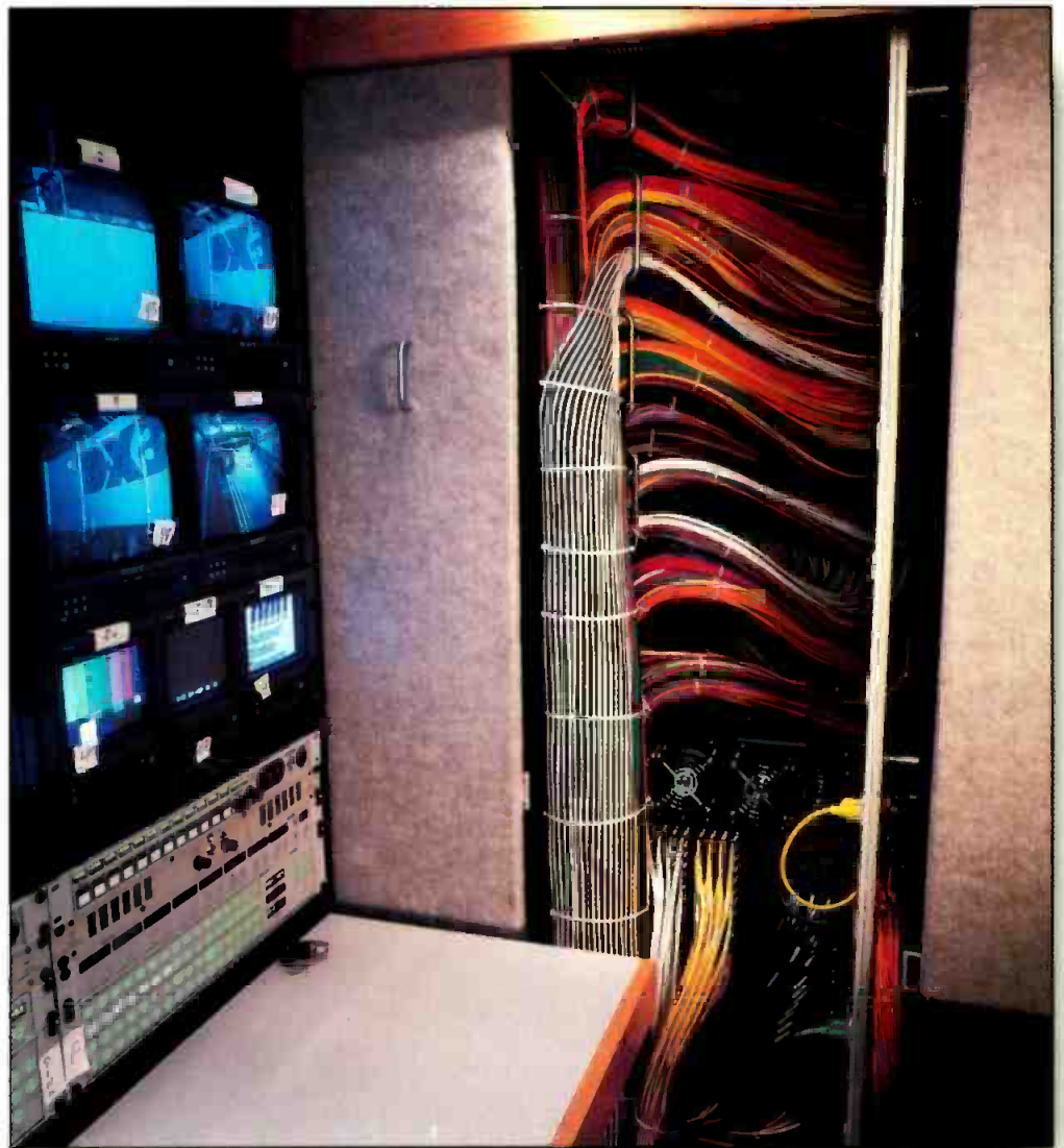
Wiring equals weight. The weight of the wire and cable used in a truck is a critical matter. A savings here can actually permit the addition of another tape machine or other critical device. Shown here is a wiring closet on an NMT truck. Photo by Concept; Deborah Rice and John Benson.
