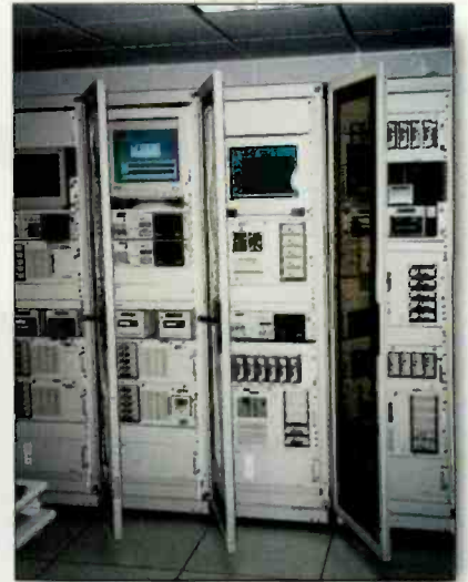
Server location is important in extending the MTBF.
