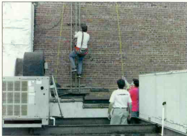
Contractors can perform specific duties more efficiently and can also help with local ordinance compliance.
