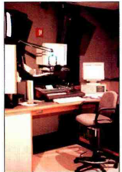
The second production room for each station uses a Yamaha O2R console.
