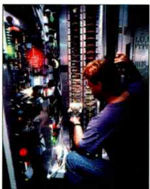
22 New developments in transmission
