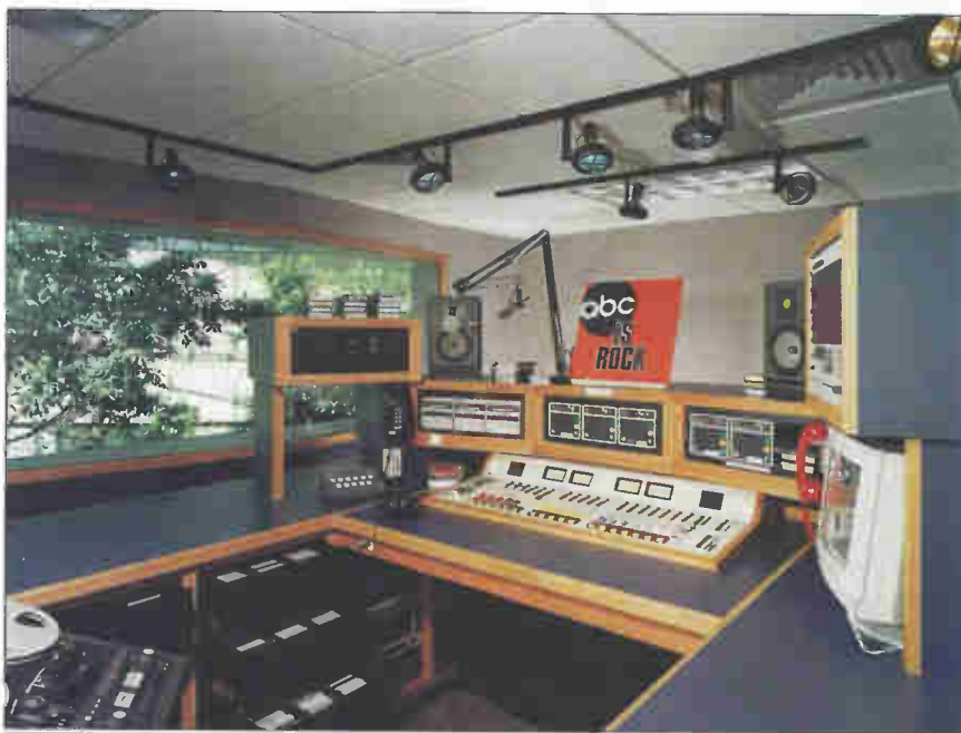
One of 13 broadcast studios in the new ABC Radio Network's headquarters in Dallas. Each studio occupies about 225 square feet, and includes a variety of digital and analog equipment. Flexible planning also allows easy future updates.
