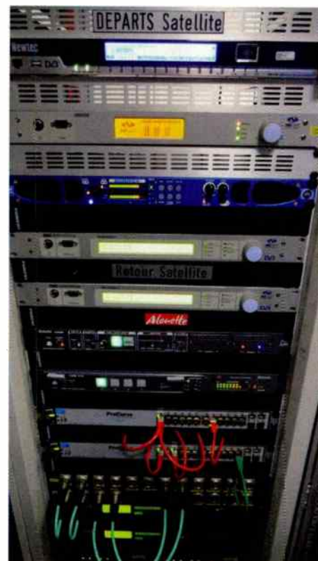
Satellite distribution equipment shown in Alouette's rackroom: uplink encoders and confidence receivers.
