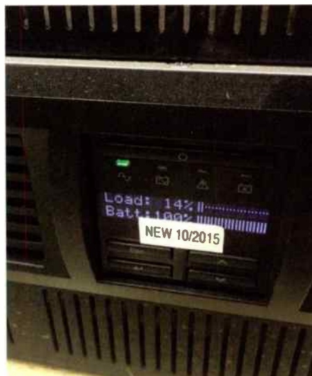
Put a label on the UPS, either when it is new or when the batteries are changed.
