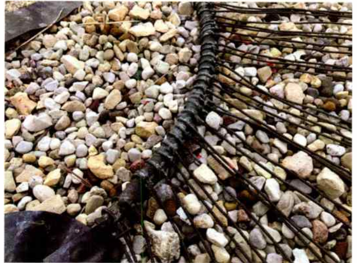
Usually, a system will have a ring and screen around the base of the tower where all of the radials are connected together. Check the integrity of this structure, including the brazed joints.
