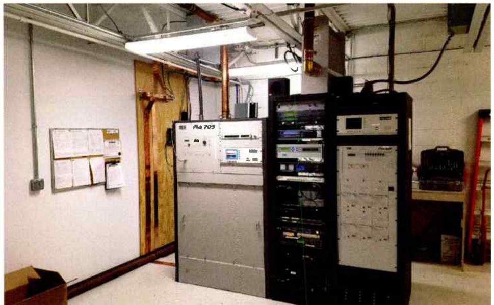
WICR(FM) uses a BE FMI-703 as the main transmitter and an FMI-201 as its auxiliary.
