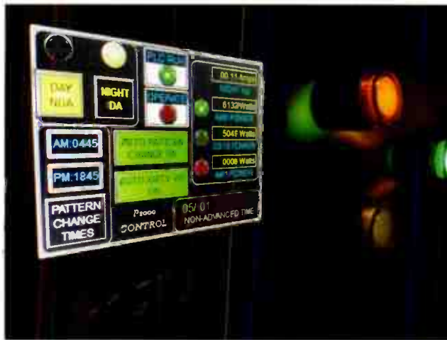
Fig. 2: Putting it all together — custom HMI designed for use with an AM directional antenna controller
