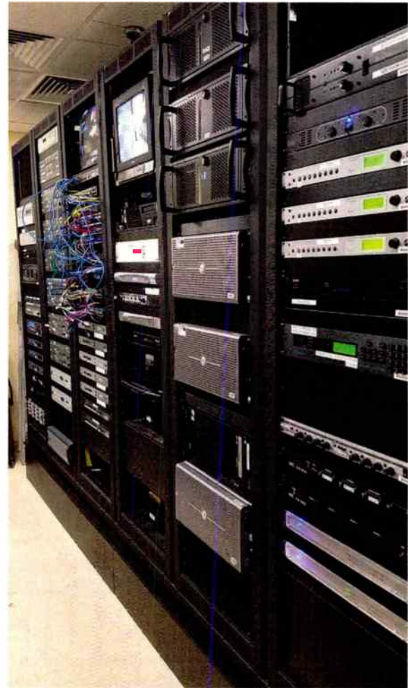
WICR's rack room, featuring Axia nodes, Dell servers, Comrex Access units.
