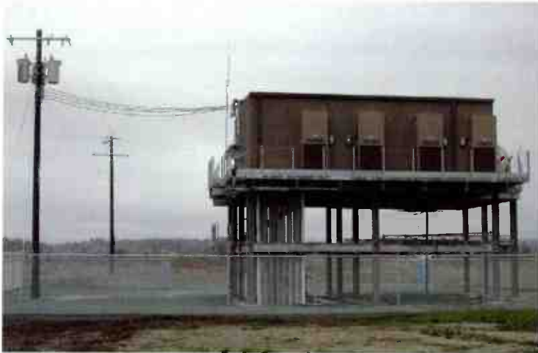
The KRKO/KKXA transmitter building was raised 16' above ground to mitigate the potential damage from flooding.
