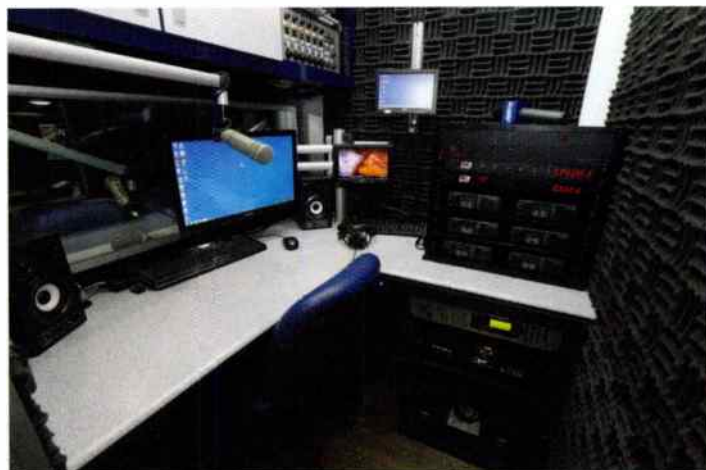
Control room 2 is also used as an editing suite.
