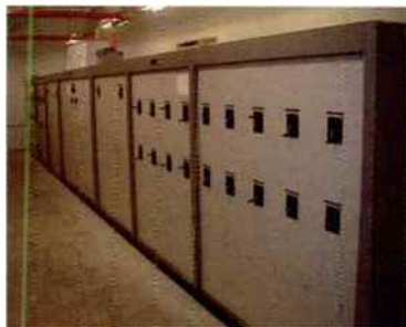
CUSTOM PHASOR INSTALLATION
