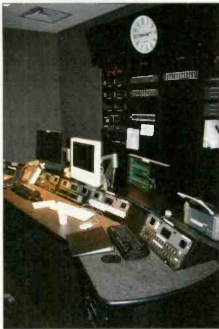
Master Control provides monitoring for various network feeds and automation systems.
