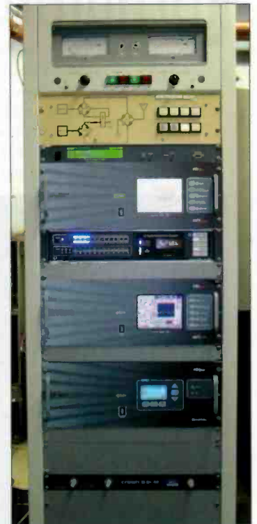
The final Harris HT\HD+ Transmitter installation
