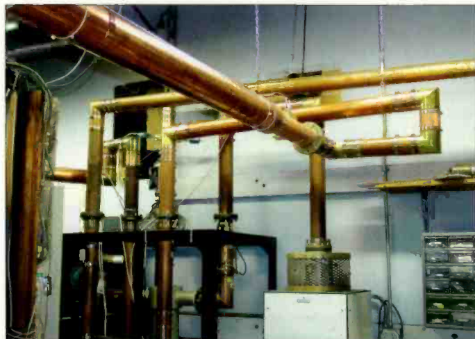
Plenty of copper and brass plumbing
