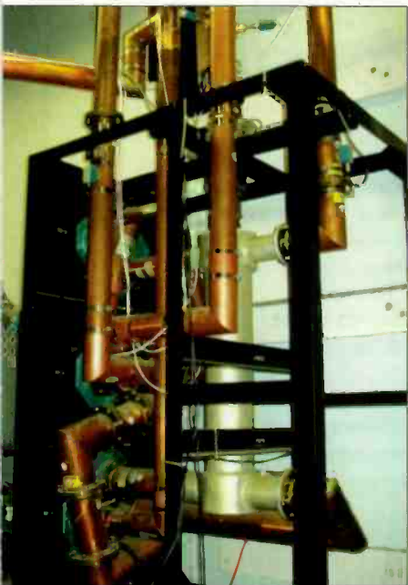
The existing Dielectric combiner switch was re-used for the HD Radio installation.
