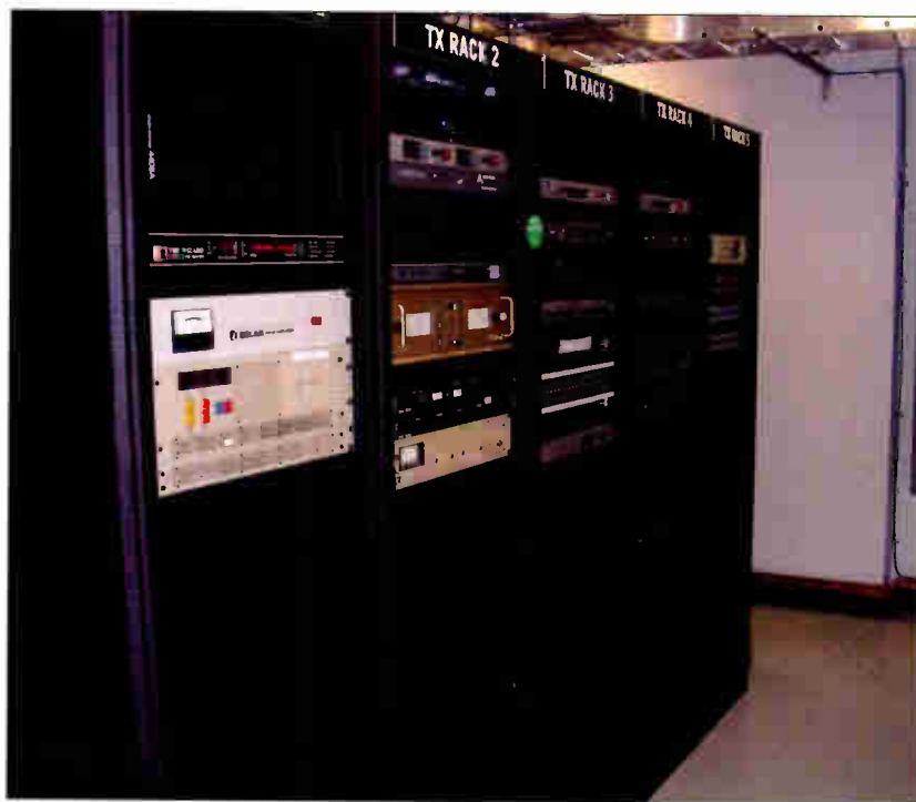
One of three rows of racks in the technical operations center.
