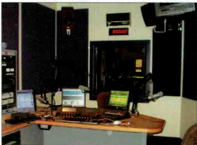
The control rooms have similar layouts. This is control room B.
