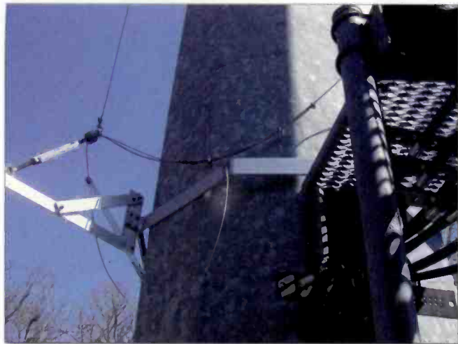
The fold wires and feed ring are shorted to this monopole tower. Typical for monopole towers, this occurred after the tower settled.
