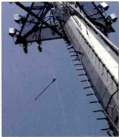
In addition to settling, regular tower wear, such as this broken stand-off insulator and loose safety cable, can affect the performance of a detuning system.
