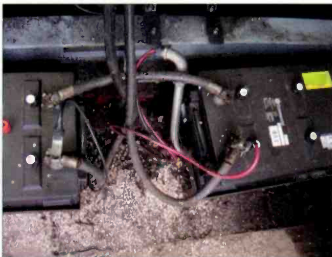
The battery connections, electrolyte and charger are simple items to check.
