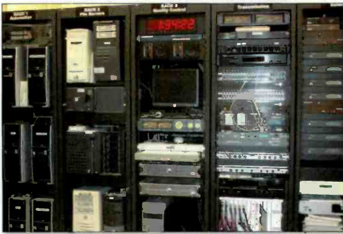
The technical operations center houses six racks.
