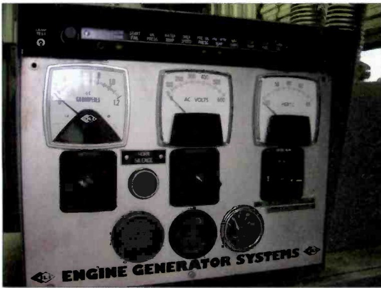
An hour meter is useful to keep detailed records of genset maintenance.
