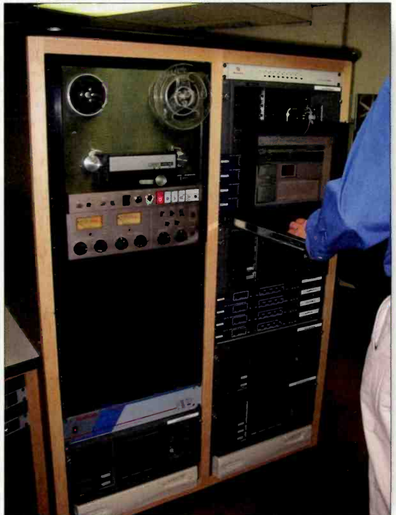
View of the equipment rack in the control room.
