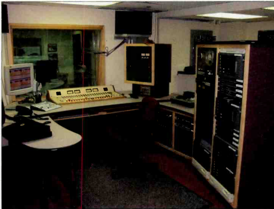
The redesigned control room at the USDA.
