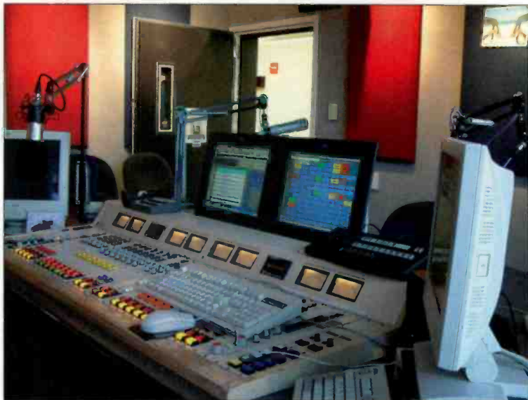
Monitors and keyboards overwhelm the BMXIII-32 console in the sports network control studio.
