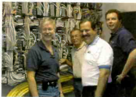
StudioHub+ wiring installed by Technet Systems', (L to R) Lindsay Collins supervising engineer, Bob Smith, Mark Blisbee with Stu Albert, contract engineer (in white) in front of the newly installed Radio Systems' StudioHub Interconnect System.
