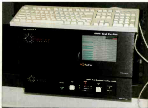
Close up of the rack-mounted IBOC exciter.
