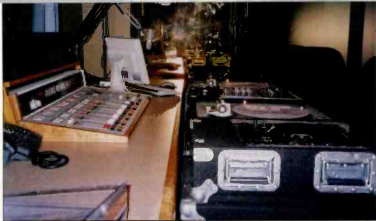
While efforts are made to standardize facilities across the company, individual station needs are still important to the facility's design.
