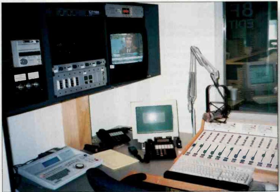
The edit suites, rooms 8F through 8I, have analog consoles with selectors for the sources on the Klotz router.
