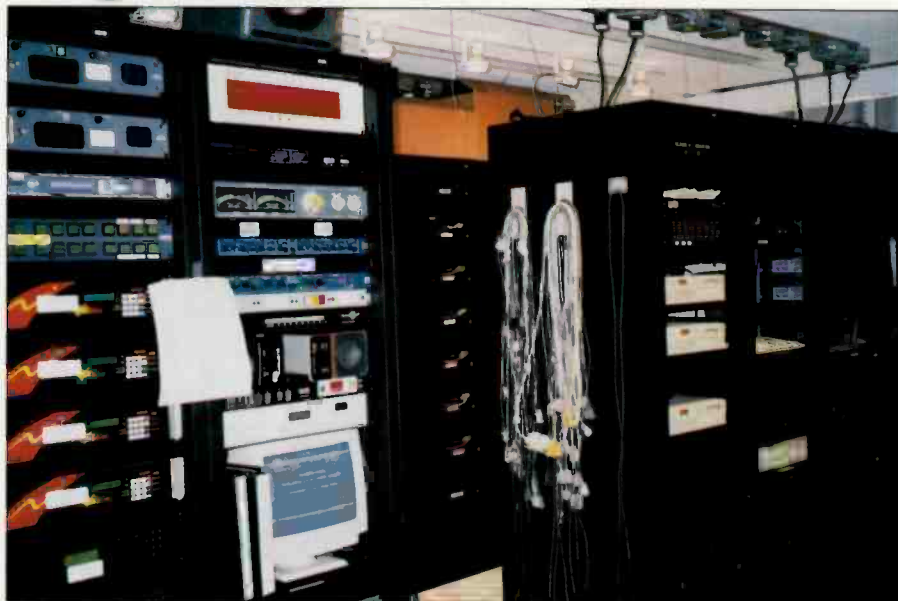
The rack room efficiently occupies the floor space at one end of the facility. The second row of racks houses the computer-based equipment.
