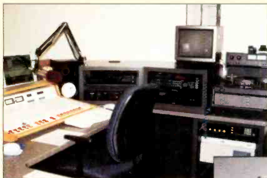
The production rooms also serve as back-up control rooms.
