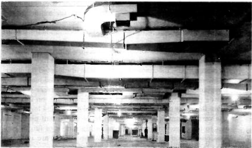
Fig. 23—Extensive overhead ducting to cool high-heat dissipating telephone equipment.
