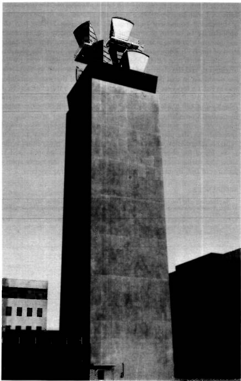
Fig. 29—Enclosed radio tower, with vertical access provisions and antenna waveguide systems, erected on an equipment building.
