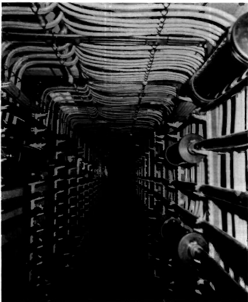
Fig. 12—A subgrade cable entrance facility with provision for cable penetration through basement walls, ceiling, and the outer wall to upper floors.
