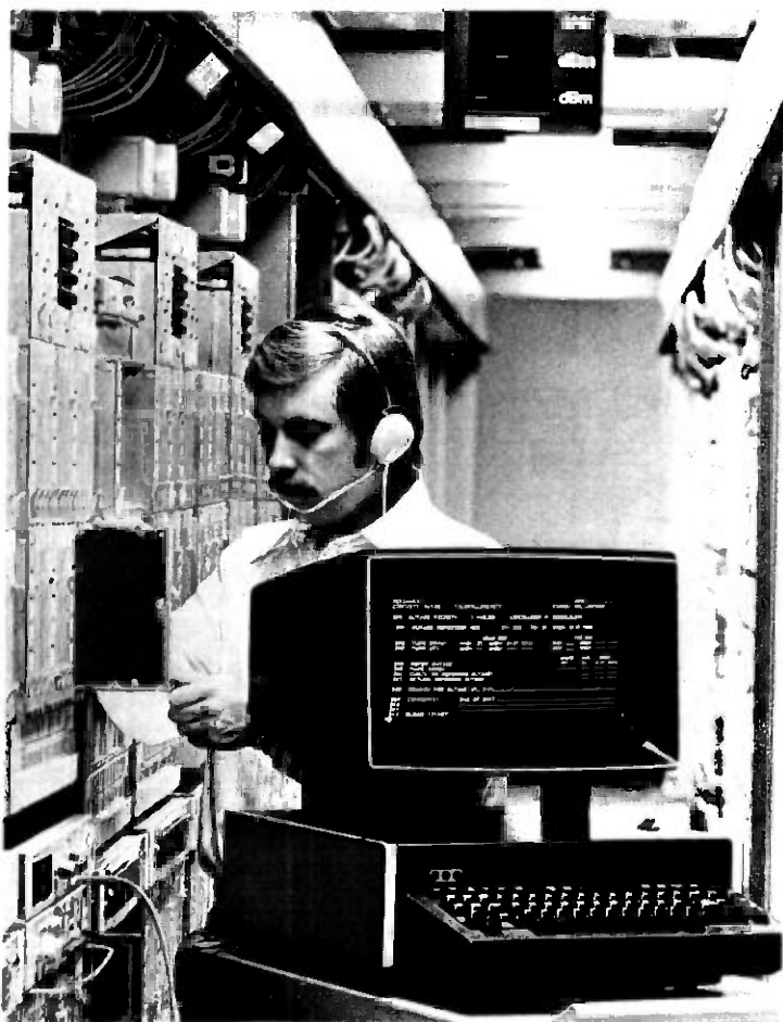
Fig. 8—Terminal Equipment Center (TEC).
