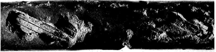
Fig. 5—Underground wire damaged by insects after two years of service in Decatur, Alabama.
