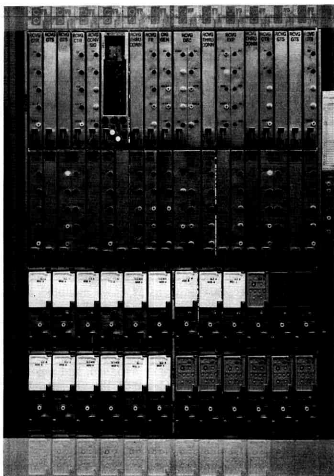
Fig. 6 — Group and channel units in place for one D1 bank.
