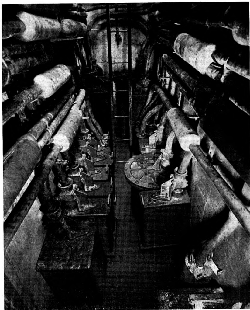
Fig. 28A—Another auxiliary vault installation of exchange area loading. One end of vault. At time of photograph, 33 cases containing a total of 11,241 coils were installed in this vault. A majority of the cases appear both in this view and in the view of Fig. 28B. 25 cases have 303, 304 or 305-coil complements, each of the other 8 cases have 455 or 456 coils. The total complement comprises 2 cast iron cases, 17 rectangular welded steel cases, and 14 tubular thin steel cases. The individual coil codes are 612, 613, 614, 622, 623, and 643. The coil inductances are: 88 mh, 70%; 135, 27% and 175 mh, 2.7%. 35% of coils have permalloy cores; the others have molybdenum-permalloy cores. 57% of coils have formex insulated windings.
