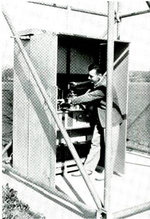
W. F. Bodtmann checking frequency of terminal equipment. Complete terminal, including power supply, is mounted in housing at base of tower.
