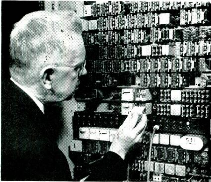
M. C. Goddard with the laboratory model of the trunk frame for switching arrangements for coin telephone dialing.
