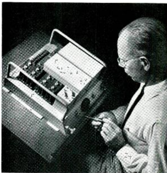
A typical rectifier, regulated magnetically, used in the "floating" storage battery. Here, the author is adjusting the degree of line compounding.
