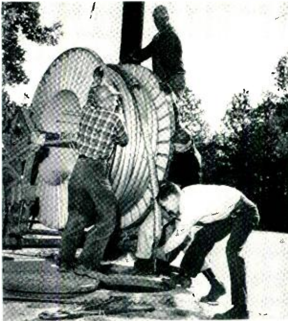
Installing a Bell System cable: with both cable and open wire, carrier systems can be applied to permit many conversations over a pair of wires.
