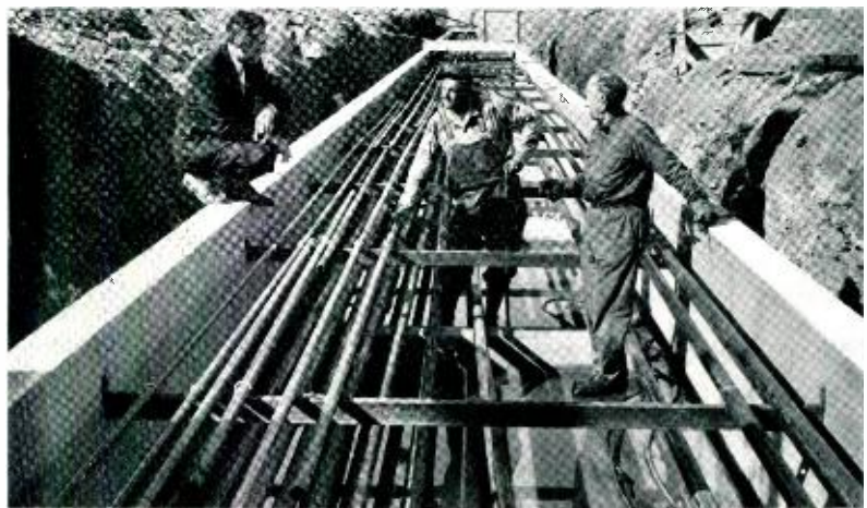
Construction work on the trough for the dry-land ocean. Trough will be covered with earth to help maintain constant temperature within.
