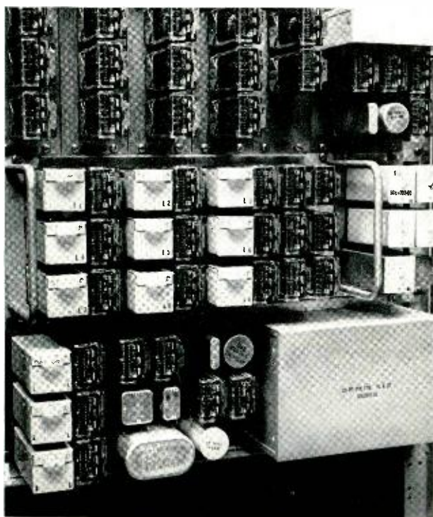
Fig. 3—Typical station-system installation for single talking link class of service with twelve stations and some associated 1A1 system equipment.
