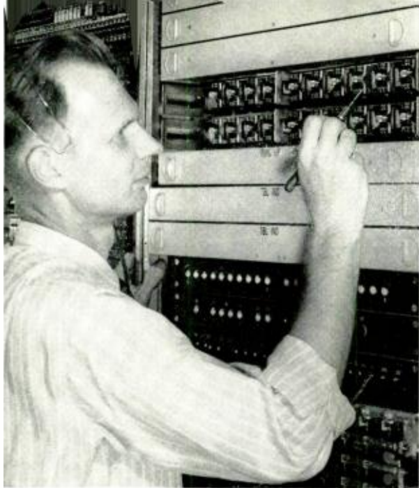
Fig. 2 — F. R. Lehman of the New York company tests relay operation in concentrator equipment.
