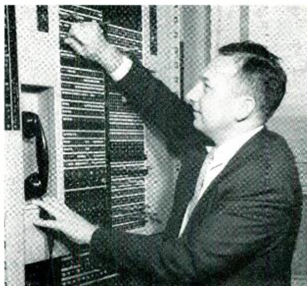
Fig. 2 — W. W. Connick makes a change in the circuits at the traffic-control lamp panel.
