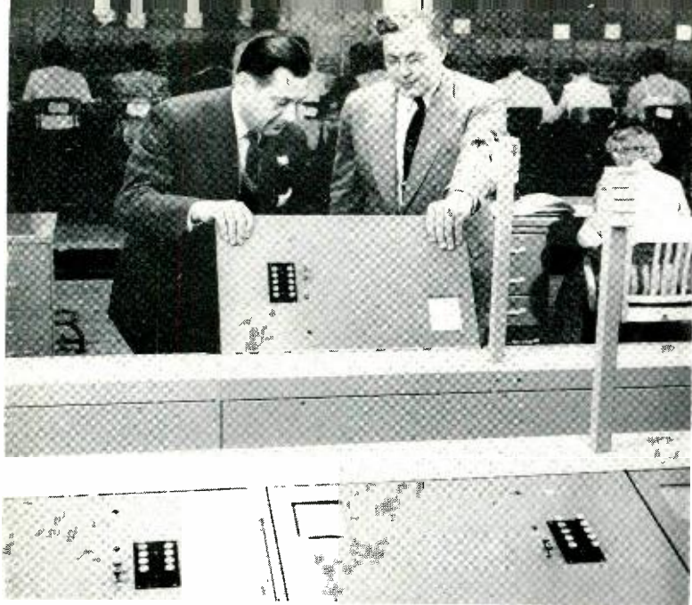
Fig. 5 — At the New York city office during installation of C.A.M.A. equipment, J. J. Cozine (right) of the Laboratories inspects operator switchboard positions with W. A. Davis, Central Office Foreman, New York Telephone Company.
