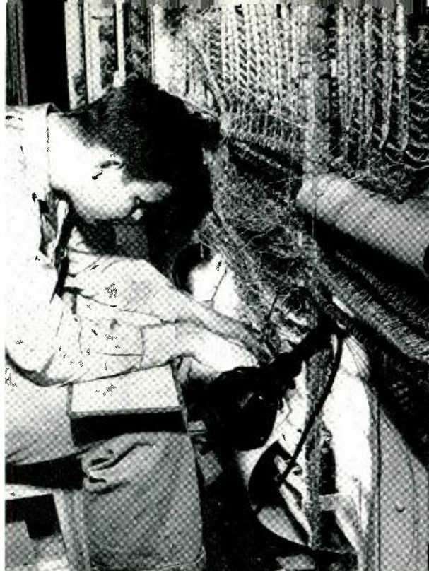
Fig. 3—Some of the cables and hundreds of wires to be changed in converting a marker connector to a decoder connector for 4A operation.
