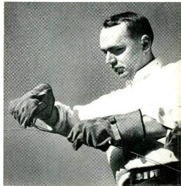
Fig. 4 — P. T. Packard demonstrates how a helically split vibration damper is placed on an open wire line prior to raising it to the insulated wire support.
