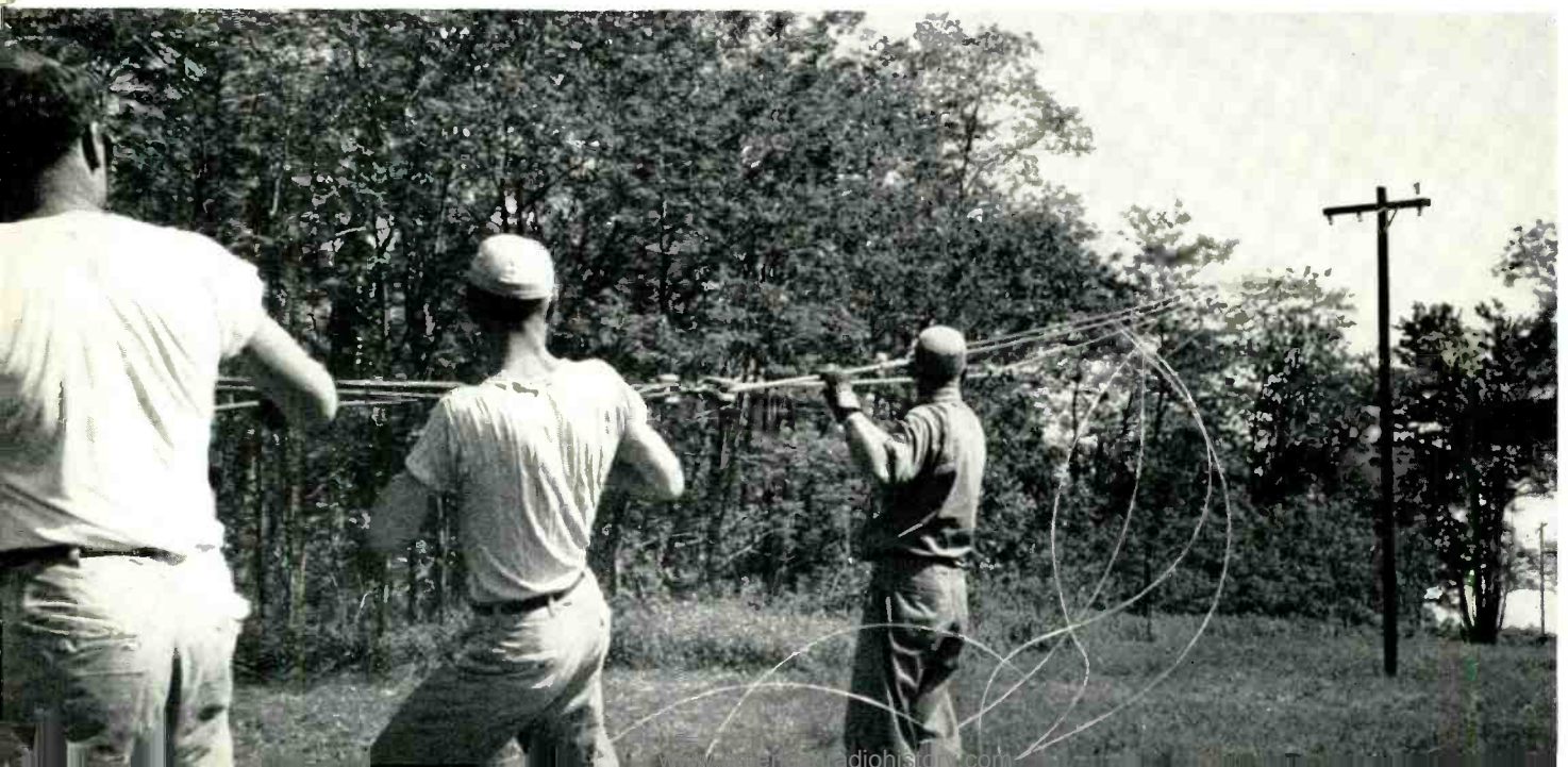
Fig. 7—Below, tensioning gear used to get correct tension in open wire lines from a ground position.
