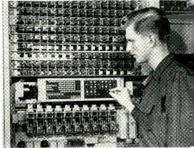
A maintenance man of The Bell Telephone Company of Pennsylvania operating the cKL key to light the lamps that display the positions of the selectors.
