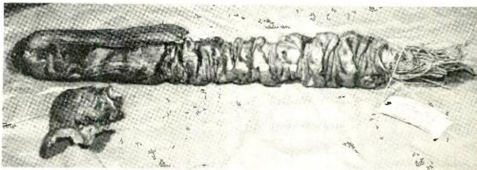
This section of a 303-pair, 19-gauge lead sheath cable recently removed from beneath a bridge was still in good operating condition.
