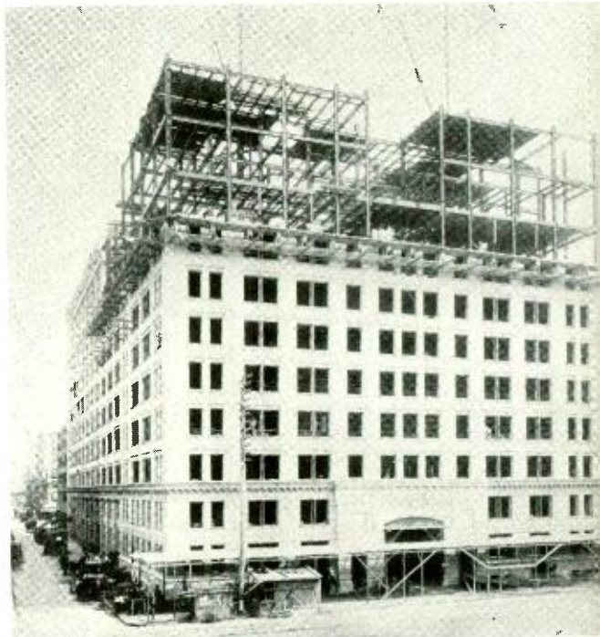
Sections A and D of 463 West Street were nearing completion shortly after the time Mary Douglas joined the Bell System
