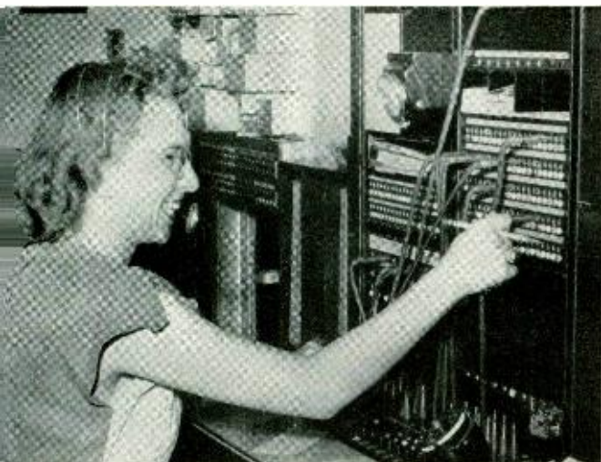
Fig. 1—Switchboard at Cheyenne Wells. Radio cabinet against the wall just visible beyond the operator
