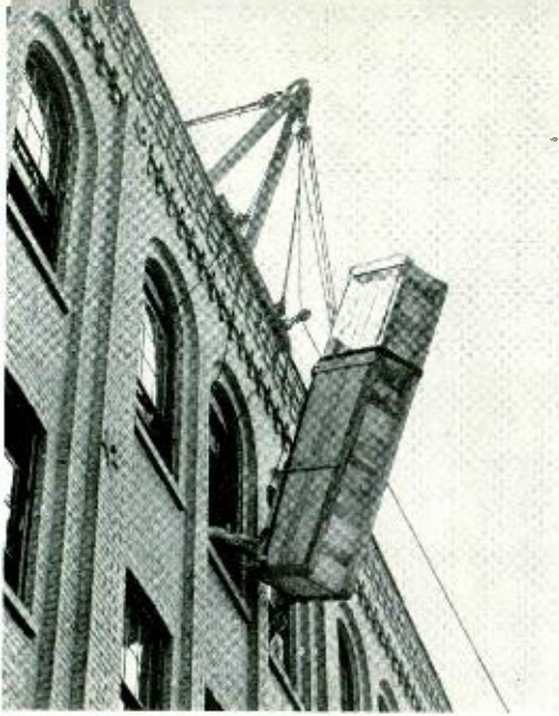
A bay of terminal equipment is swung out of a window in 4-1 for shipment to a point on the New York-Boston radio-relay circuit. The bays were built by the 4-1 Assembly and Wiring Shop under the immediate supervision of Jack Acker
