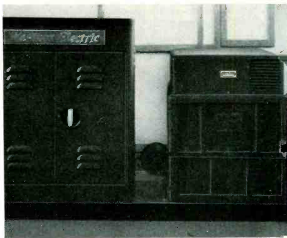
Fig. 2—Synchronizer and transmitter cabinets in the after end of the chart room
