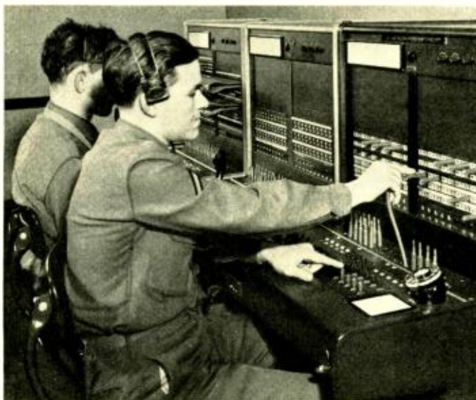
Fig. 1—Civilian Air Raid Warning Board in foreground; beyond are the test and patch boards
