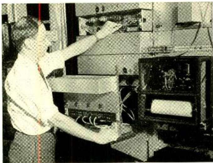
Thermistor-controlled twist repeater and temperature recorder used on laboratory trial of new type-K carrier system over the cable recently installed on the roof of Section R at Bethune Street. J. P. Kinzer is changing one of the connections on the repeater
