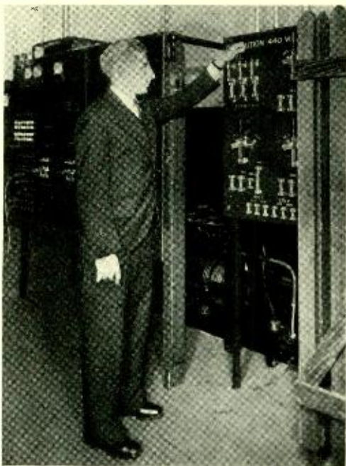
Fig. 1—The transformer with its control panel, at the right of the main switchboard, is enclosed as a matter of safety
