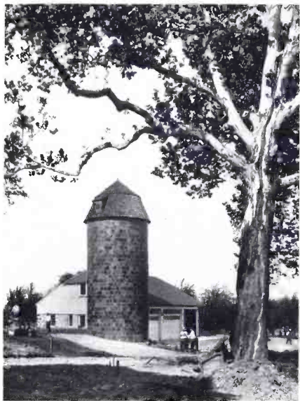
Fig. 1—Building the road to the new garage at Mendham. This building utilizes the stone walls of the old barn
