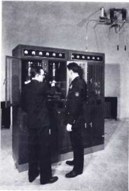
B. R. Cole, who supervised the installation, points out interior details of the new police transmitter to Patrolman Edward Barth.
