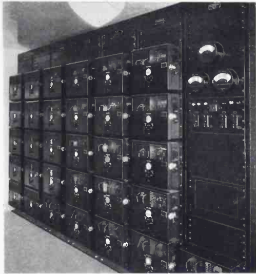
Thirty-one power amplifiers raise the level of the program for transmission to guest rooms, public rooms and distant broadcast stations. At the right is the remote control rack for the alternating current power equipment
