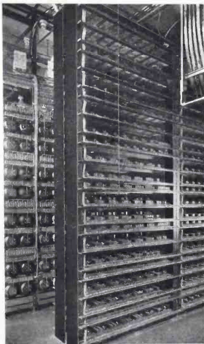
Fig. 7—Two forms of mounting were used for the older coils: on horizontal shelves and on vertical panels
