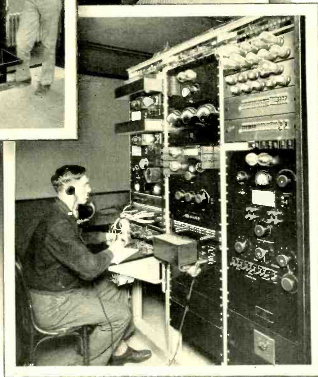
Top, the shore transmitter now at Deal which will eventually be moved to Ocean Gate, New Jersey; left, the shore receiver which is housed at Forked River, New Jersey, and H. W. Powers and C. Breunich of the Long Lines Department; bottom, C. F. P. Rose of the Radio Research Department and the line terminal equipment, enclosed in copper screening at Deal
