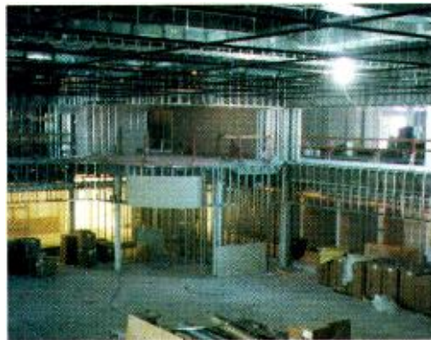
The interior of the new Miramar, Fla., facility is still a work in progress.
